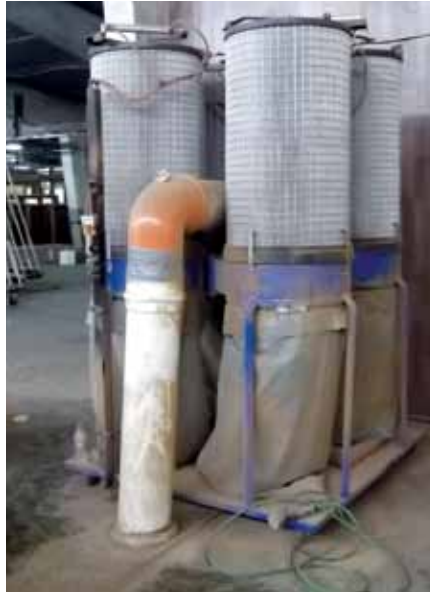
Before modernization 15 mobile dedusters have been overstrained
